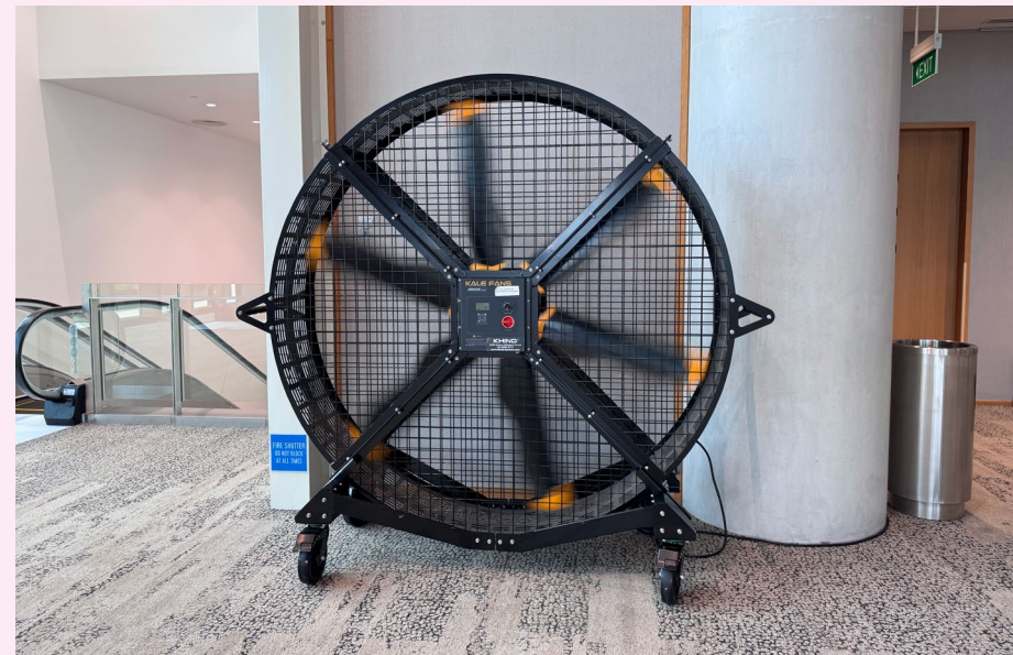
Hybrid cooling system introduced within SCCC premises
